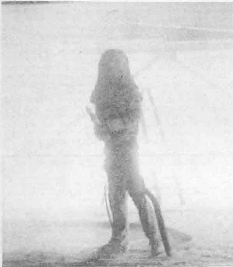
TAKE ME TO YOUR LEADER: A repairman sand-blasting one of UMSL's parking garages last month was an alien sight on campus. The garages, which had not been extensively repaired in years, were given a complete overhaul [photo by Earl Swift].
